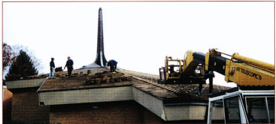
Removal and stacking of the roof tile. Photo Courtesy of Pfister Industries, Inc.
