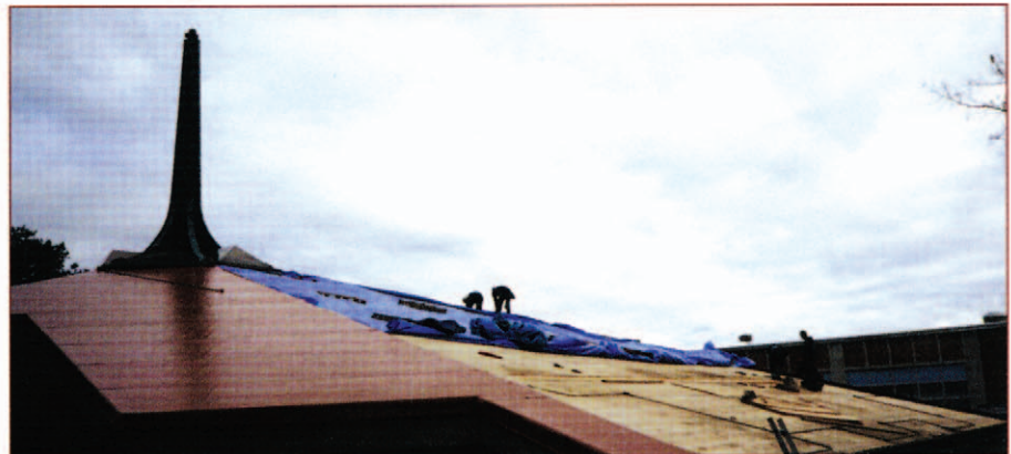
Application of the terra cotta field membrane. Photo Courtesy of Pfister Industries, Inc.
